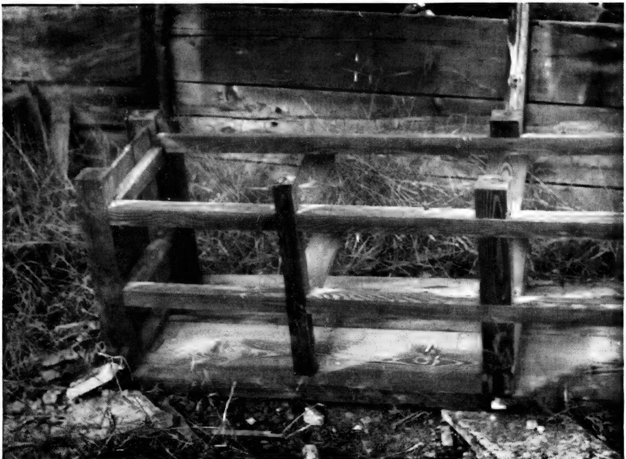
Photo No. 22. NAGASAKI. Timber framing scorched by heat radiation at \frac{1}{4} mile from the centre of damage. The surface is unscorched where it is shielded by the uprights. See paragraph 52.
